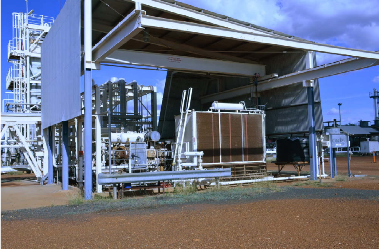
Photo 1- The Kincora Gas Plant is located south-west of Wallumbilla in Queensland. Gas processing at the facility commenced in 1977. The plant also produces LPG, condensate and crude oil and has a storage facilities within the Newstead Field. Current gas processing capacity is estimated at 25 TJ per day and is connected to the Wallumbilla Gas hub which in turn provides a route to the southern, Gladstone and Brisbane markets.
